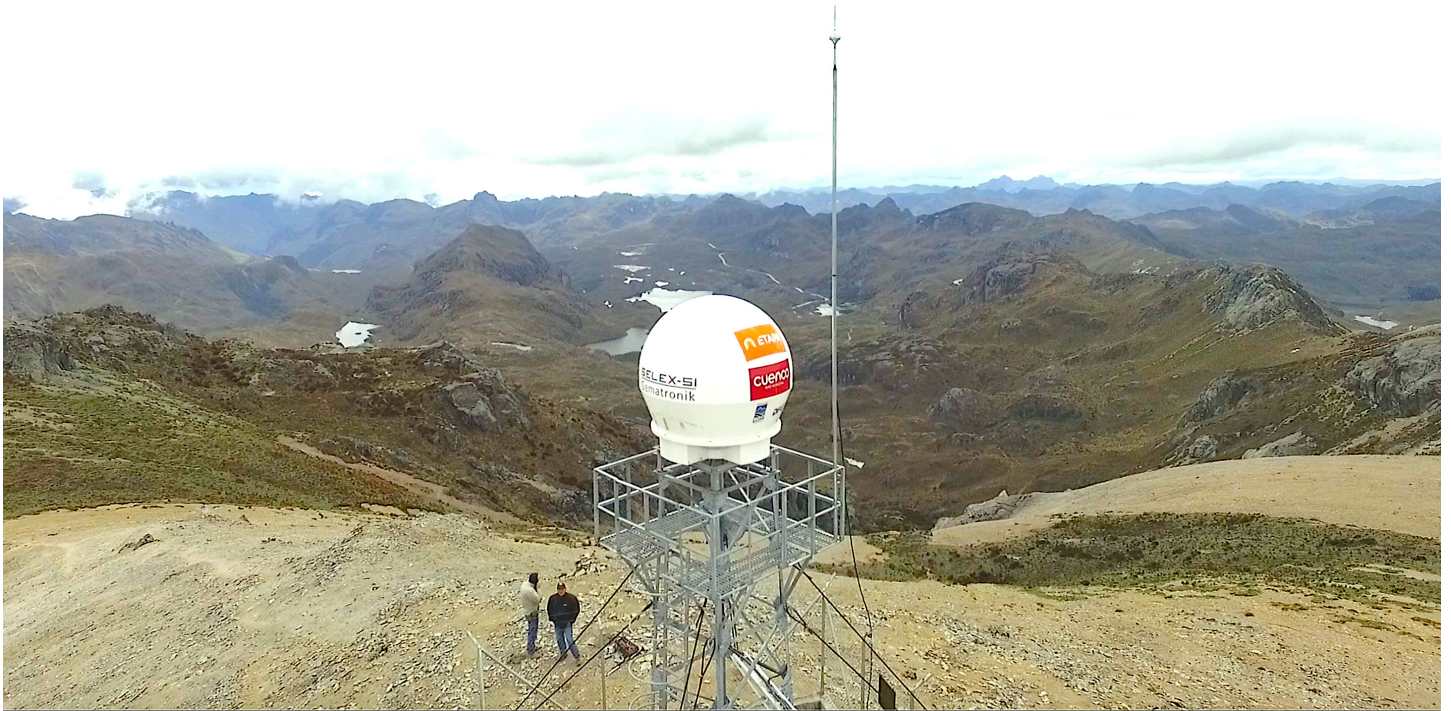
Figure 2: X-band Weather Radar (CAXX) located at 4550 m a.s.l at the West of Cuenca. Photo: Snapshot of Empresa de Telecomunicaciones, Agua Potable, Alcantarillado y Saneamiento de Cuenca (ETAPA EP) video
